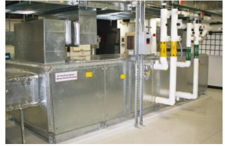
The general-service air-handling system used for the tests. It serves the classrooms, offices, and common areas of the Energy Resource Station with a nominal capacity of 7,800 cfm.
