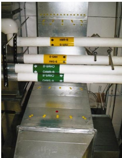
A floor-up view of the supply-air ductwork, showing the direction of air flow from the fan discharge. Traverse Plane Nos. 1 and 2 are in the vertical section of the ductwork, while Traverse Plane No. 3 is in the horizontal section.
