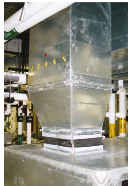
The vertical portion of the main supply-air ductwork of the general-service air-handling system. The yellow duct plugs identify Traverse Plane No. 1.
