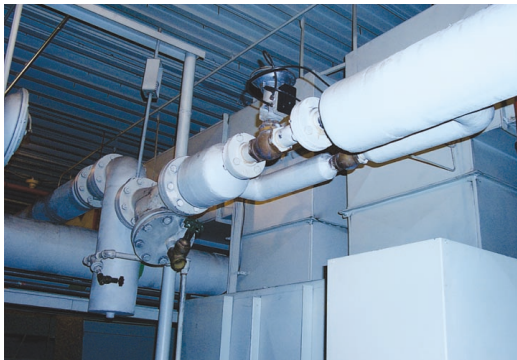
A steam-control valve with reducers.
