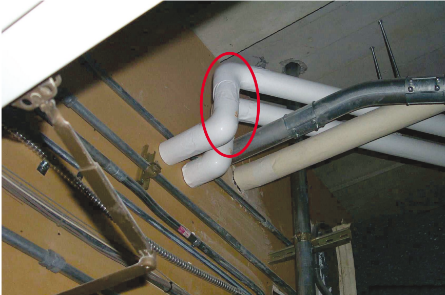
PHOTO C. This 10-in. change in the elevation of return piping trapped a large slug of water upstream, flooding the load. The untrapped elevation change in the parallel steam line (behind the return line) caused condensation associated with achieving and maintaining the supply-main temperature, creating waterhammer in the system.
