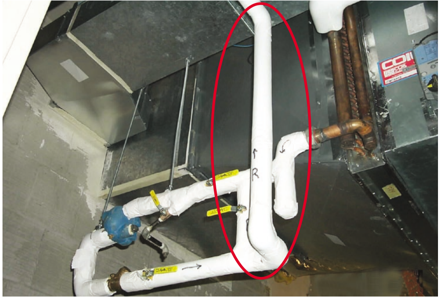
PHOTO D. This modest (less than 2 ft) change in the elevation of return piping from a steam reheat coil creates a condition that sees the coil flood until the reduced heat-transfer surface causes the steam valve to open and introduce steam at a pressure high enough to blow the condensate up into the elevated return main. This sudden change in available heat-transfer surface causes an excessive supply temperature, which results in cycling and instability. This coil was equipped with a vacuum breaker. However, that only guarantees that the coil always will be at or above atmospheric pressure and that it will drain somewhat predictably to a gravity return system. It cannot cause the condensate to flow uphill.
